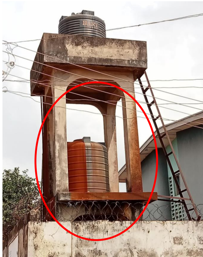
Figure 1.6: Evident water contamination in water tanks
